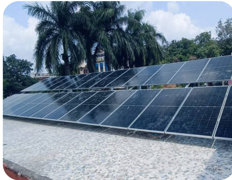
Solar power plant installed at Wagar Seva Sansthan
