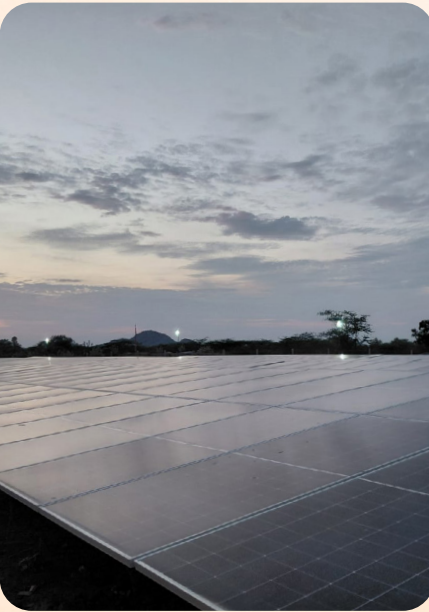
Twilight over the plant Site: Choudhary Renewable Energy Pvt. Ltd., Jalore District
